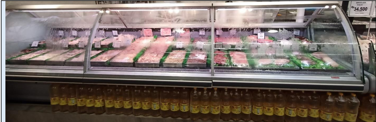
Above: fresh meat counter in an outlet of a major supermarket.
